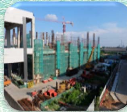
Project Pure DC (Data Center)
